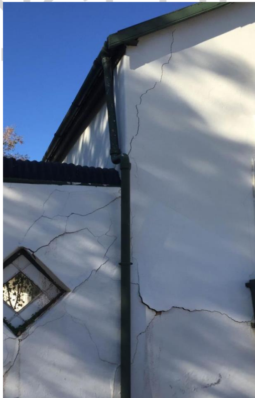
Damage caused by water ingress
