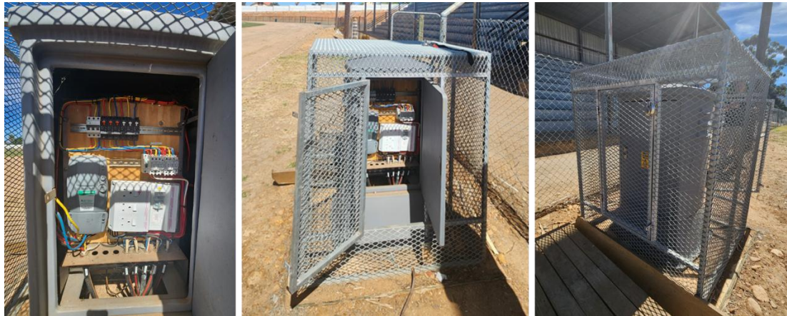
Figure 2: Sample of light control box with HDG steel cage
